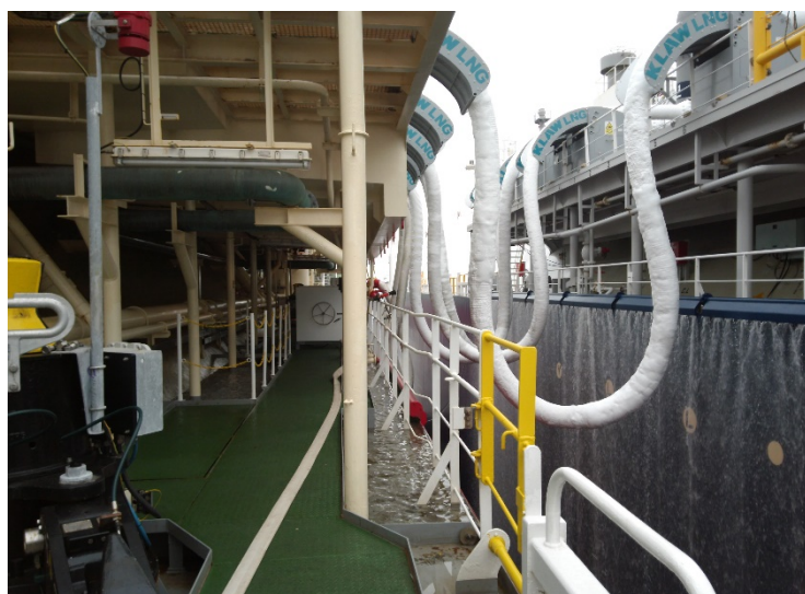
Figure 34 Water Curtain / Deluge
