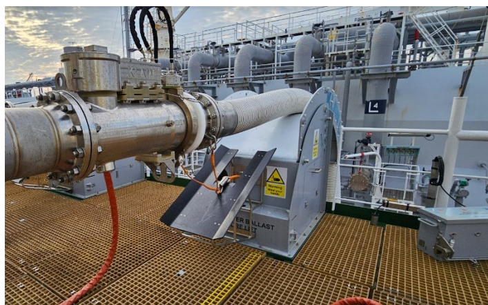
Figure 17 Fall Arrest system on the FSRU
